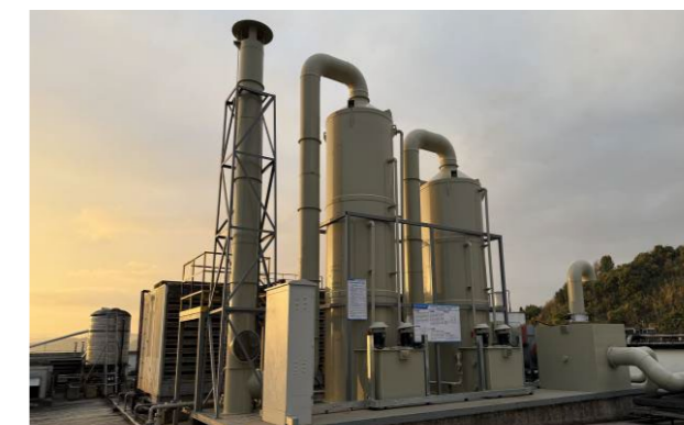
VOC Treatment System for Extraction Tower
