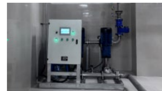
Reverse Osmosis Brine Reuse System
