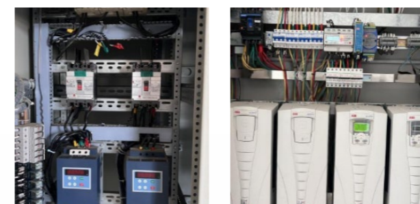
Electrical control cabinet before (left) and after (right) the optimization and retrofit
