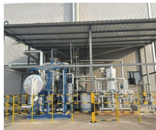
Condensate waste heat recovery system
