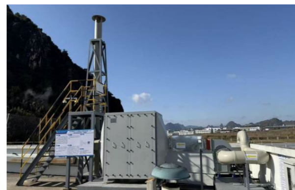
VOC Treatment System for Underground Tank Farm
