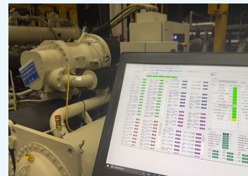
Application of Intelligent Testing Technology for Chillers
